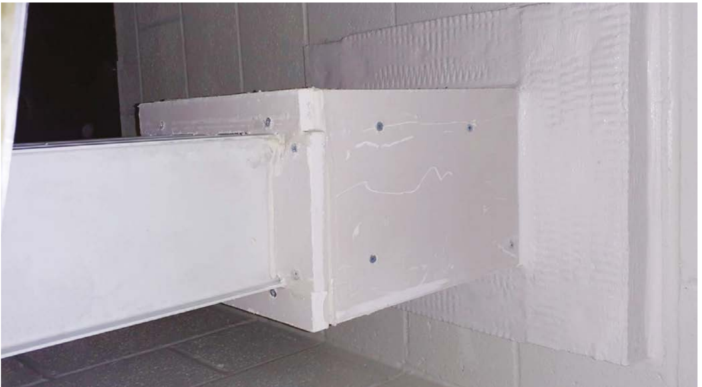
Figure 1: Insulation fitted to busbar electrical services.
